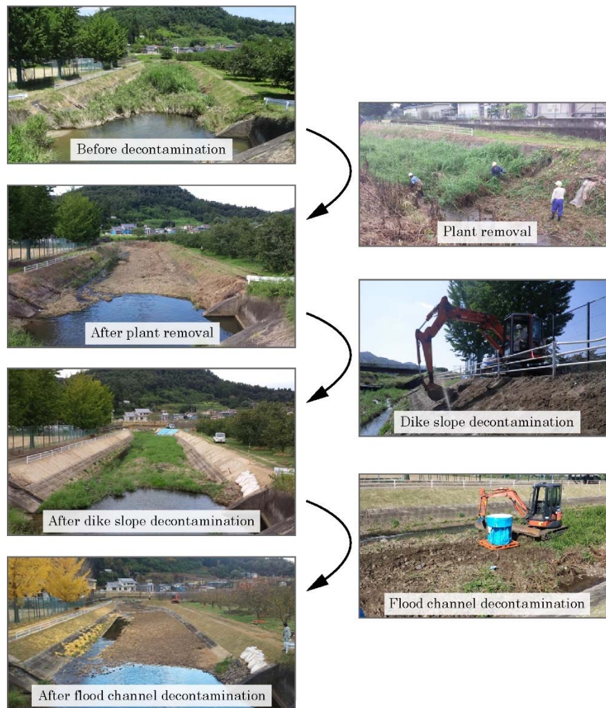
Figure 2: Photographs of the decontamination test procedures.
